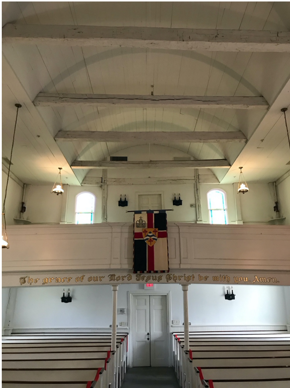
Barrel ceiling uncovered in 1937. Beams revealed are original 18 th century white oak
